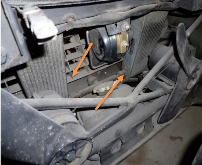
2 external engine oil coolers (fan motors and black round item in picture is not correct) S/N 9605
