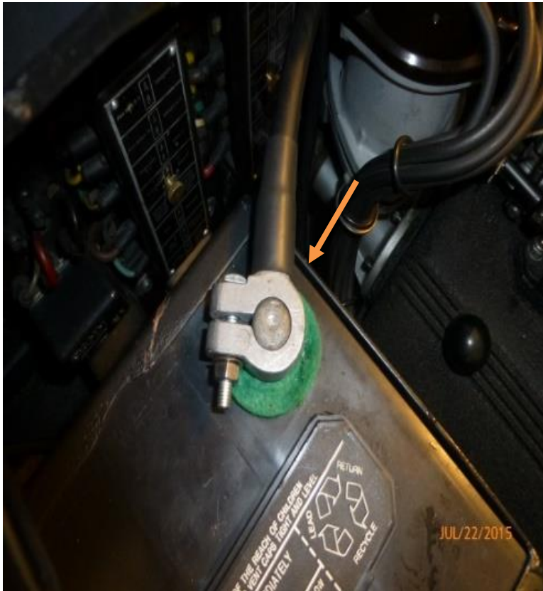
Right angle battery cable termination
