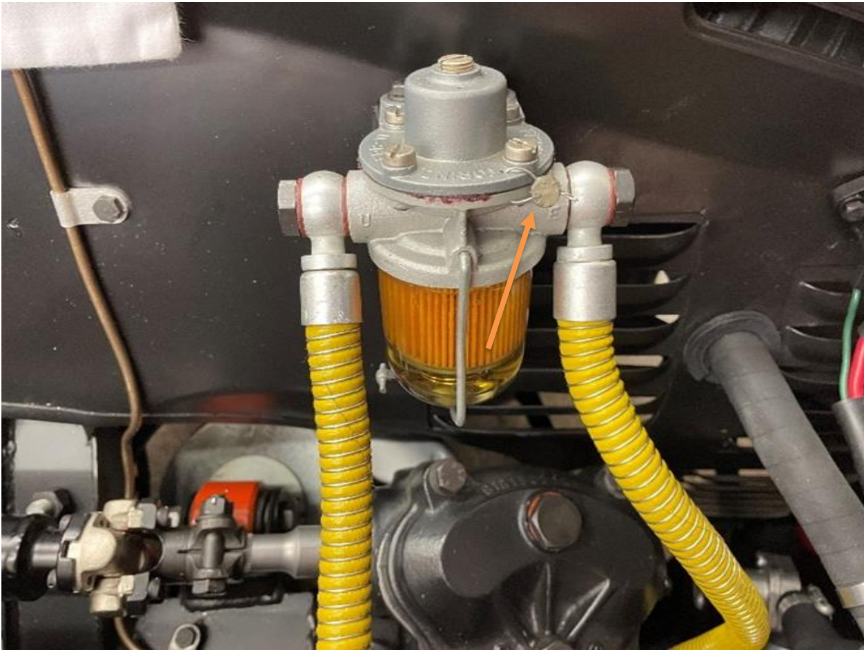
FISPA filter with hole and lead tag
